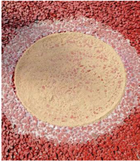
Fig. 3. The site clogging.
